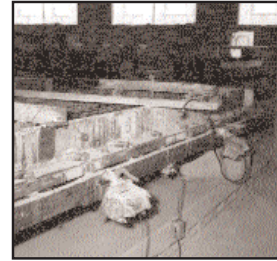
US-900 with Wedge Bracket on precast mold
